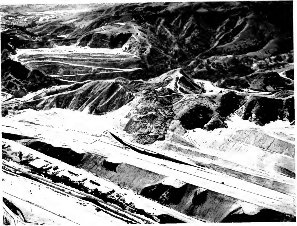
Photo 2. Earthquake-triggered landslide along the unfinished southbound lane of the Golden State Freeway, San Fernando Pass area. Weak, fine-grained, clastic beds in the Towsley Formation lurched parallel to the strike of beds and slid down along the dip (see photo 3). Failure took place during first strong shaking. Flat area in left background is a Los Angeles County sanitary land-fill. View is southwest. Photo courtesy of the Grading Section of the Los Angeles Department of Building and Safety.
